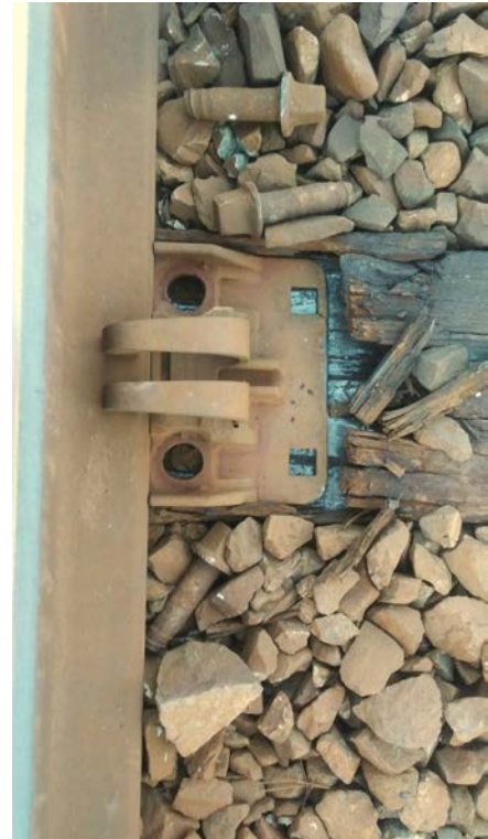
Image 1: Image of broken bolts that allowed rails to go wide, causing wide gauge.
